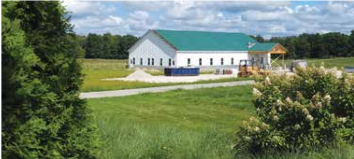
Framing and roofing of the Sunshine Training Center were almost complete before the tornado struck.
